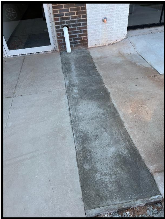
Trench filled in for the sidewalk. PVC pipe is shown coming from the wall into the trench.
