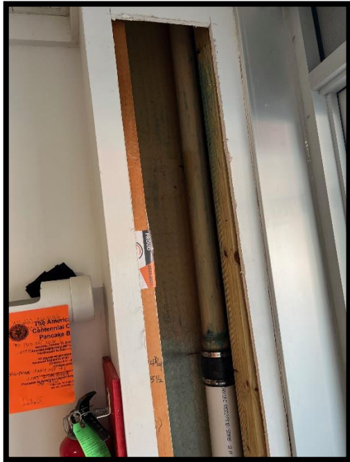
Water pipe from roof inside the wall at entryway.
