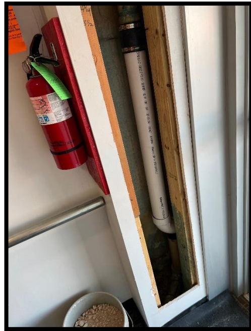
PVC plastic pipe attached to the pipe from the roof and then outside.
