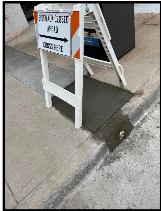
Finishing touches on the trench was to add the cement to the area next to the curb. Stan and Jim Rutledge finished the Job.
