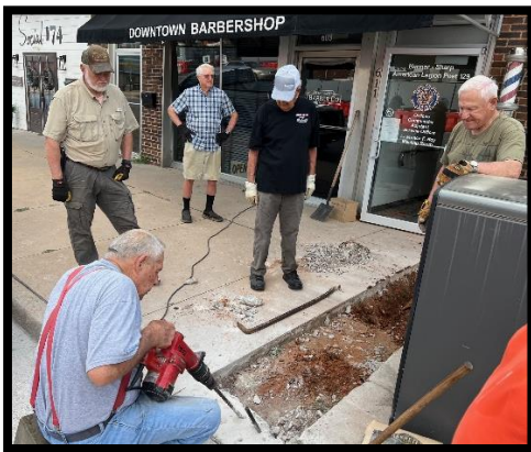
Jim Rutledge, Jim Mote, _____ and Norman Filtz wait for Stan to get the last concrete and curb out of the trench.
